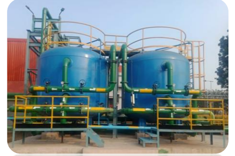
SIDE STREAM FILTER
