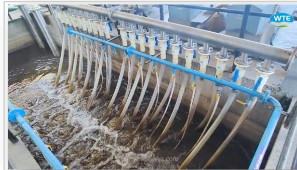
MBR STP Plant
