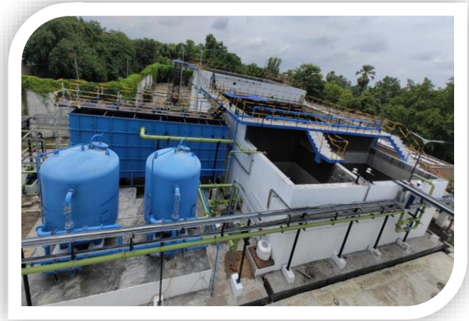
CONDENSATE POLISHING UNIT
