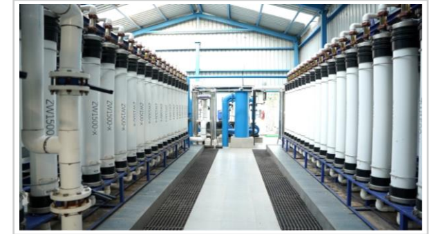
Ultra Filtration Plant
